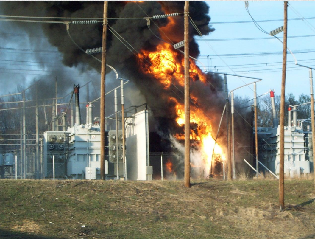
500 kV Transformer Failure in 2000
