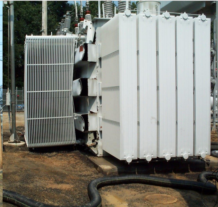
230 kV Transformer Failure in 2001
